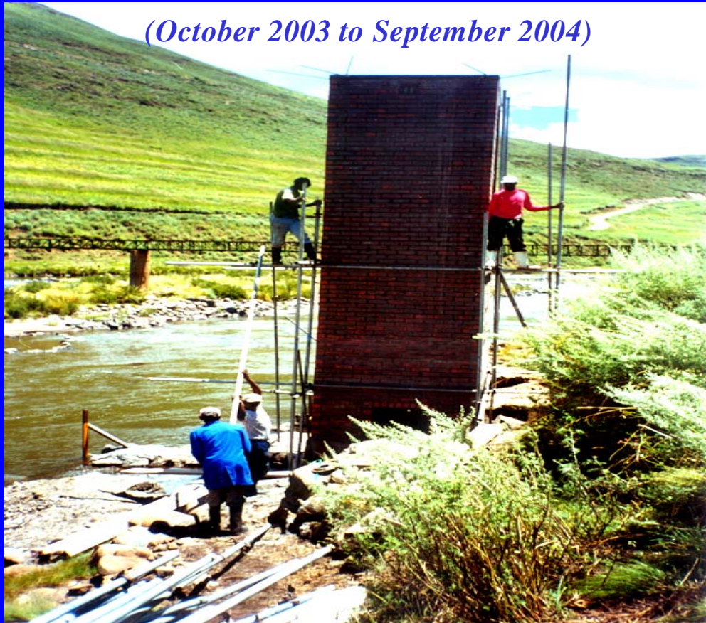
TOWER ON MALIBAMATSO RIVER @ KAO
