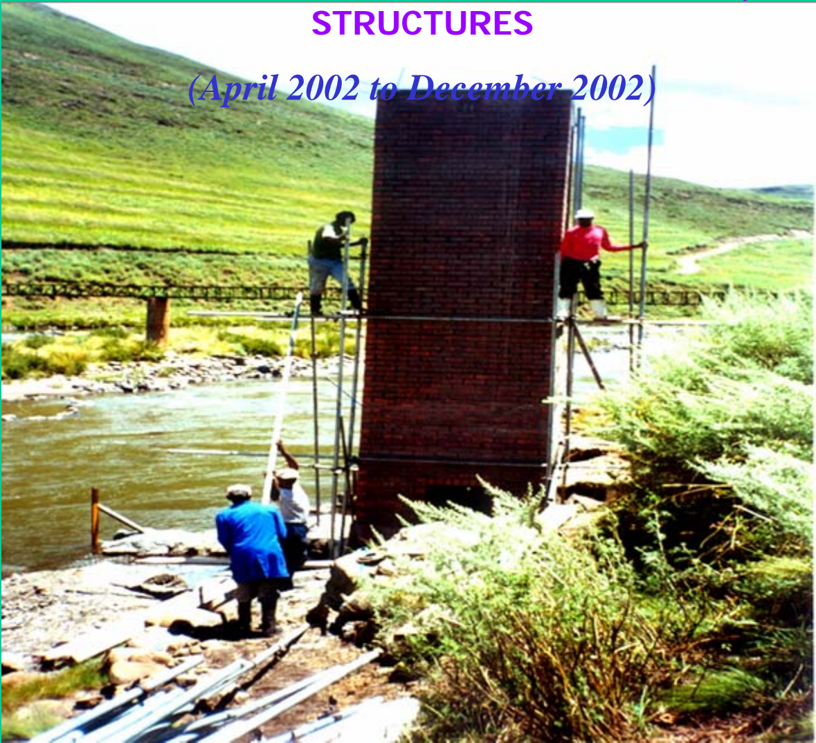
TOWER ON MALIBAMATŠO RIVER @ KAO
