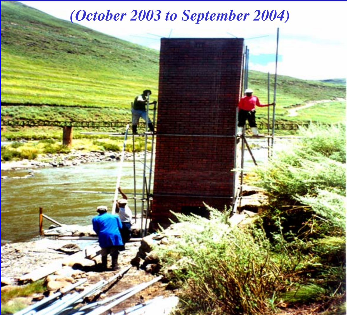
TOWER ON MALIBAMATŠO RIVER @ KAO
