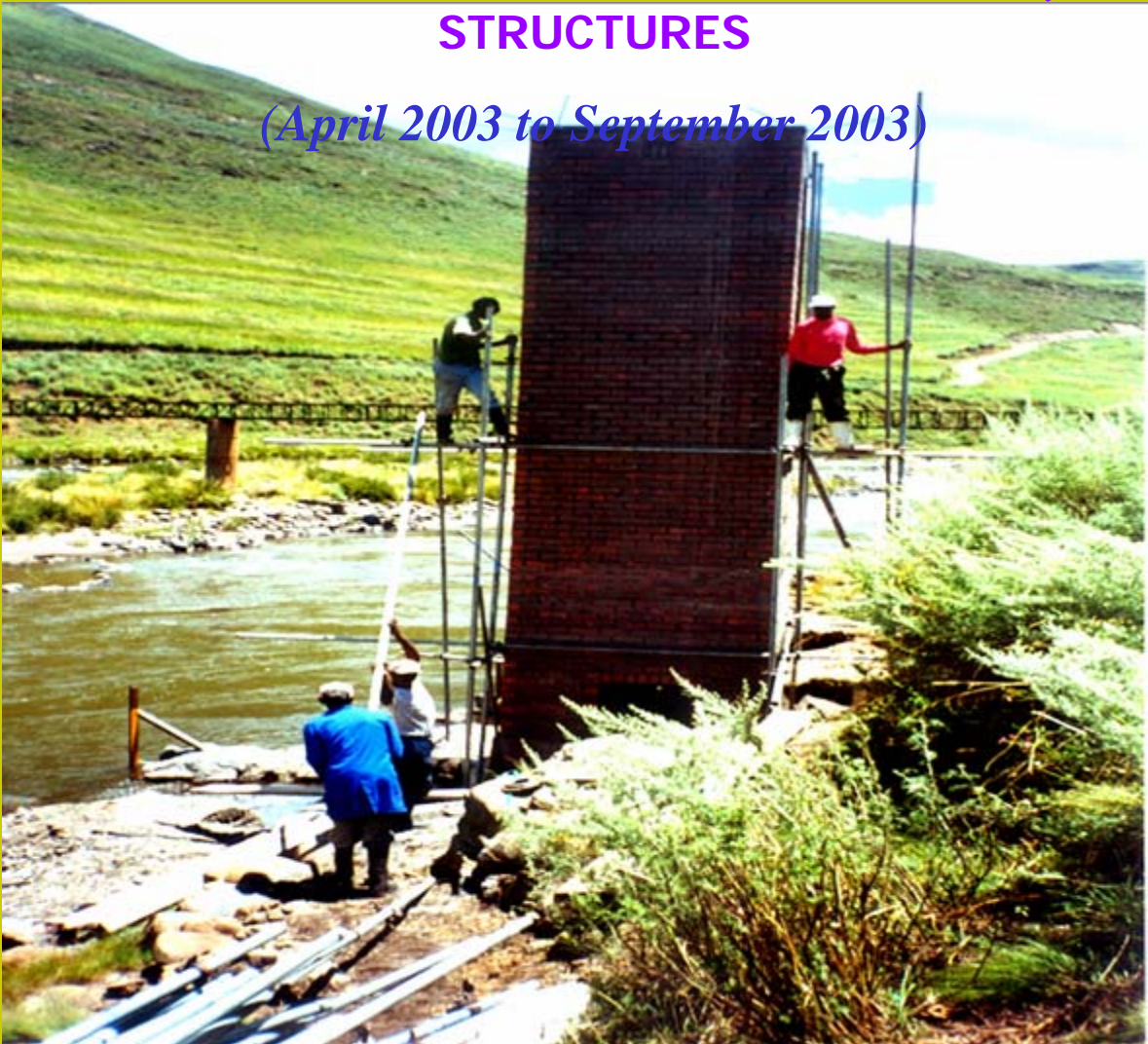
TOWER ON MALIBAMATŠO RIVER @ KAO
