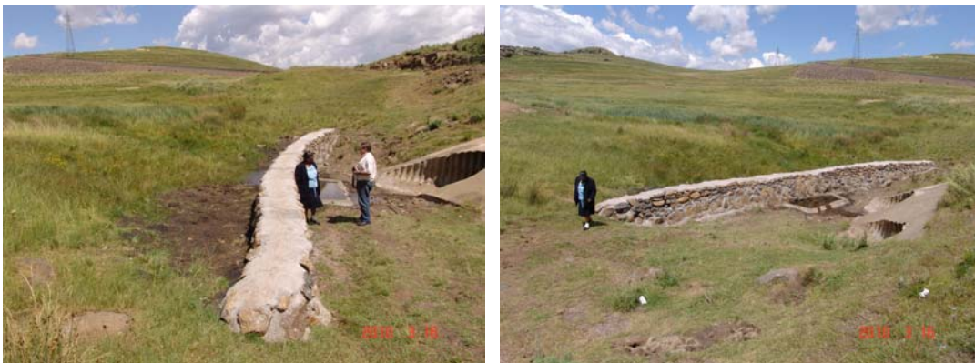
Exhibit 4 Weir at culvert on tarred feeder road to Mohale tunnel inlet. The purpose is to raise the base to which erosion is working, and prevent headward erosion into the wetland upslope. Over time sediment might build up behind the weir, in which flood flows could divert and scour around the weir. In this case extend the ends of the weir into the banks, and raise the left and right ends so weir is lowest at centre. The pond at the base of the weir is a drinking trough for livestock.
