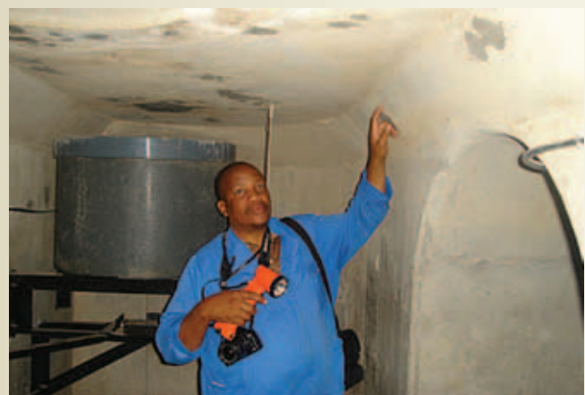
Gallery M flooded to height > 2m
