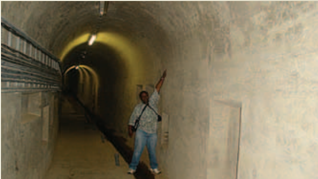
Flooded Electrical Cables
