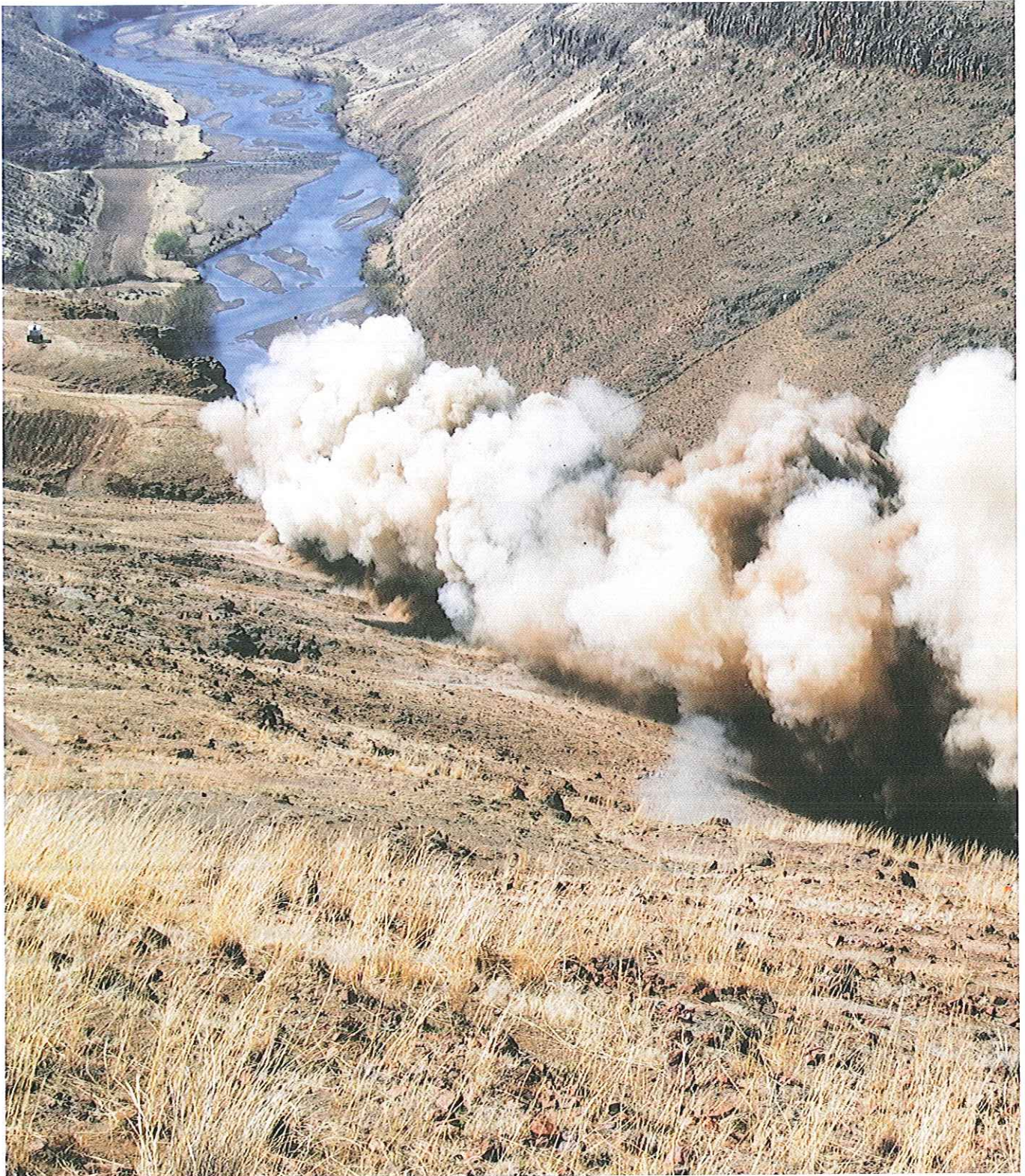
BLASTING WORKS ALONG THE SENQU RIVER IN PREPARATION FOR THE CONSTRUCTION OF THE 3.8KM LONG ACCESS ROAD TO POLIHALI MEASURING WEIR.
