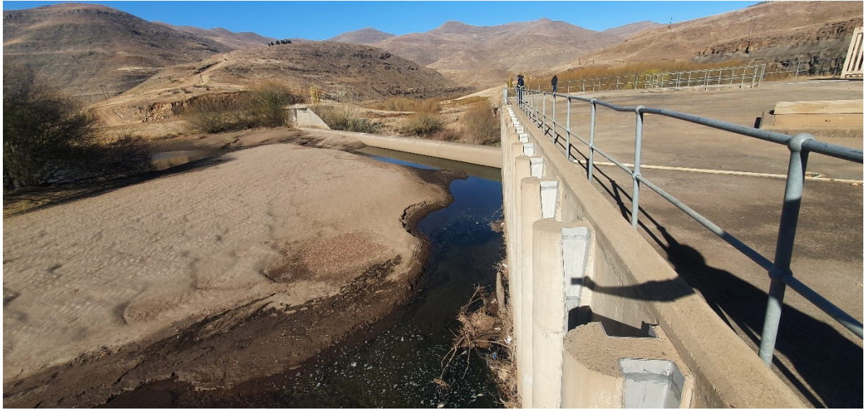
Figure 16. Sediment buildup in front of the inlet structure and weir. Hand rails are installed around the platform for safety.
