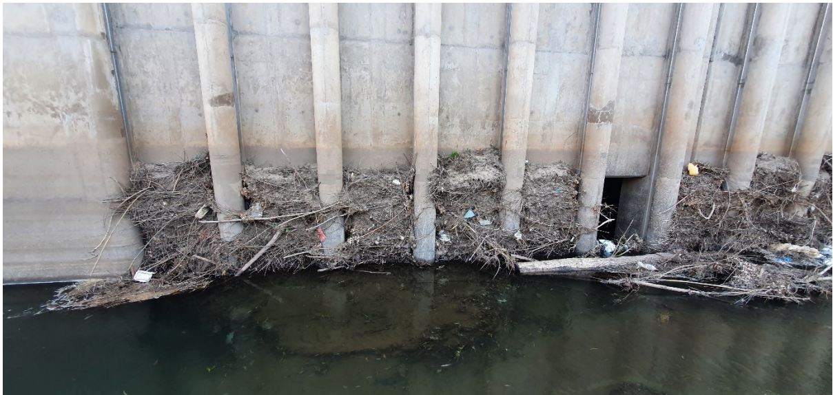
Figure 9. Densely compacted debris on the screens
