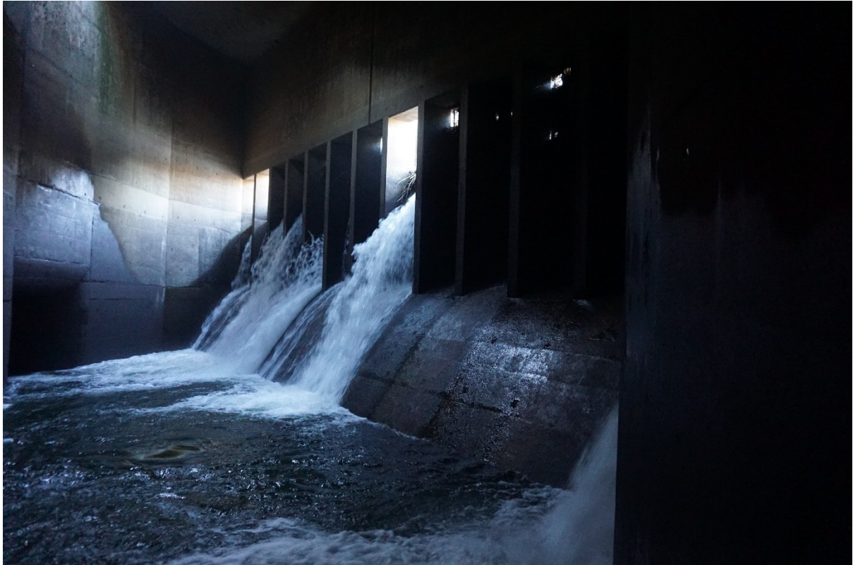
Figure 10. Inside the intake structure. The divergent tunnel is on the left. On the right are the thirteen screens. Some screens are completely blinded.
