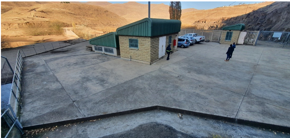
Figure 1. Panoramic view of the intake structure roof slab and parking area (7 June 2022)
