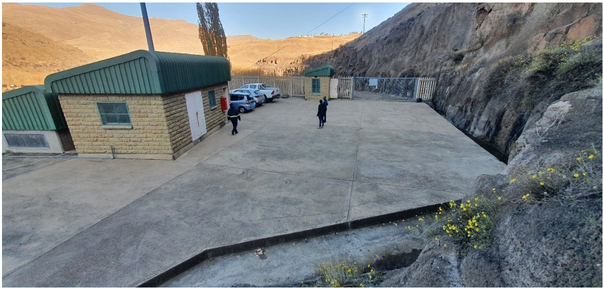
Figure 6. Entrance and access to the roof slab of the intake structure as viewed from the right bank. The roof slab is only accessible through a gate next to a guard house which is visible in the top right of the photo. The building provides access into the intake structure.
