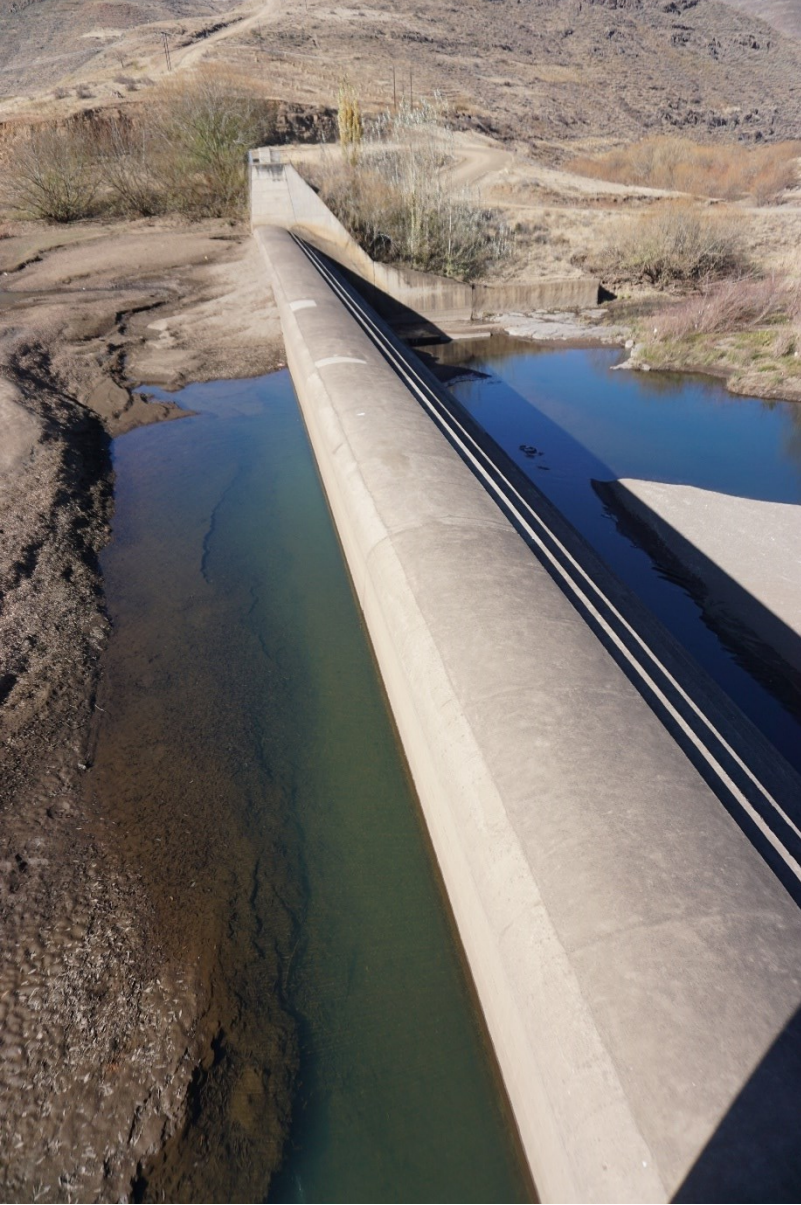
Figure 15. The ogee weir as viewed from the roof slab of the intake structure
