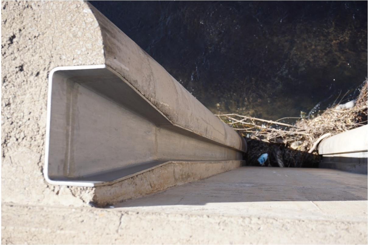
Figure 14. The screen guide channels as viewed from the top of the roof slab. The guides taper at the top.
