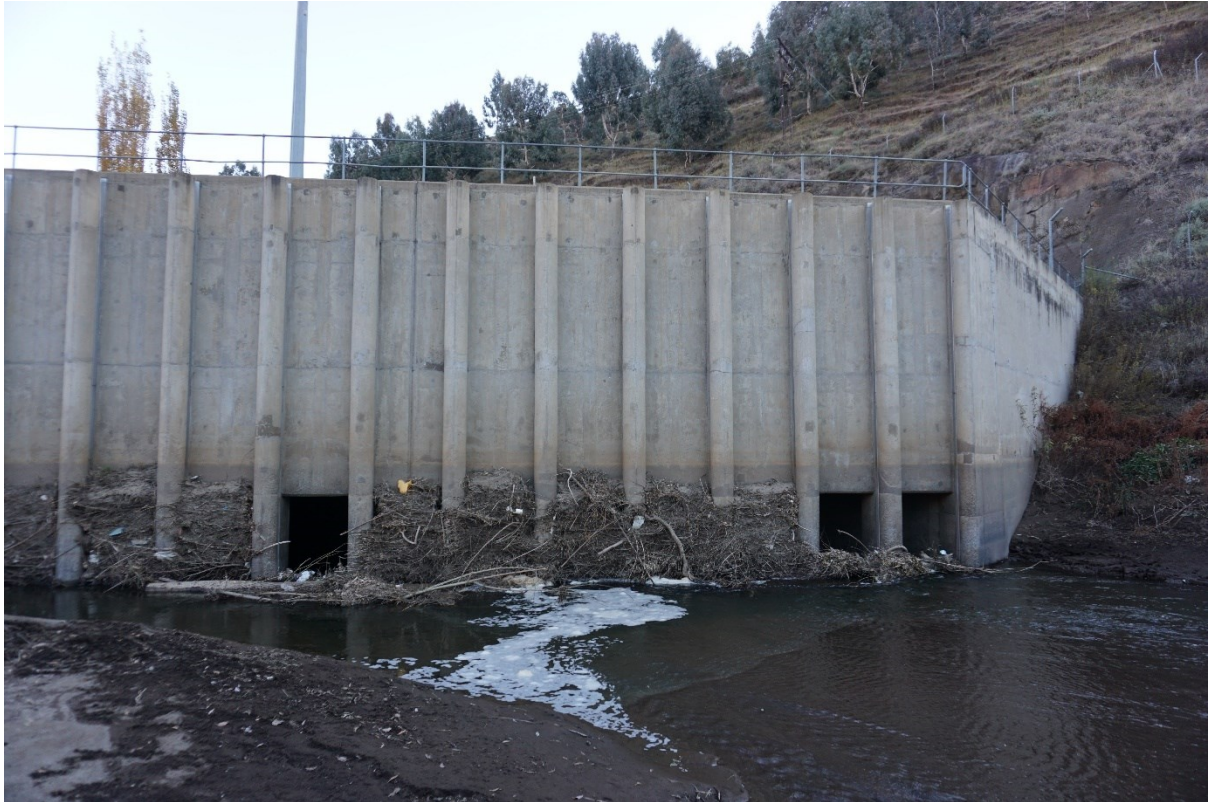
Figure 8. The intake structure as viewed from the river where sedimentation buildup has occurred. Flow through the screens is completely restricted by densely compacted debris with the screens of three screen bays removed to allow flow into the intake structure.
