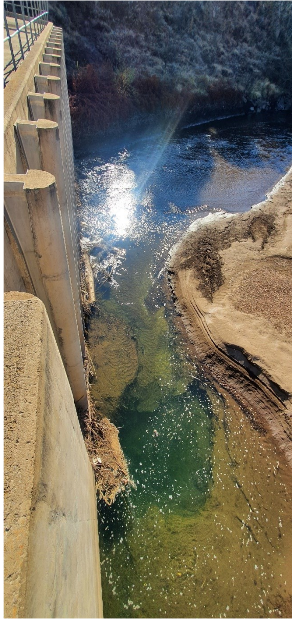
Figure 7. The intake as viewed from above. Sedimentation buildup can be seen at the intake
