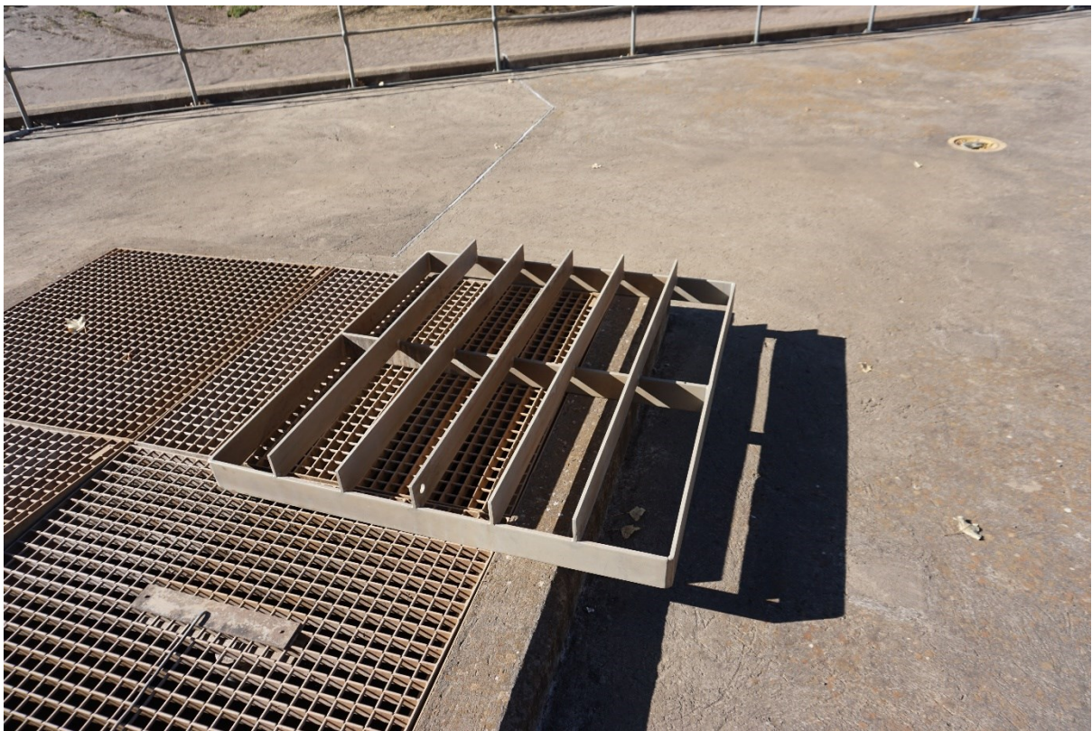
Figure 11. One of the screen panels that had been removed and placed on the roof slab of the intake structure.
