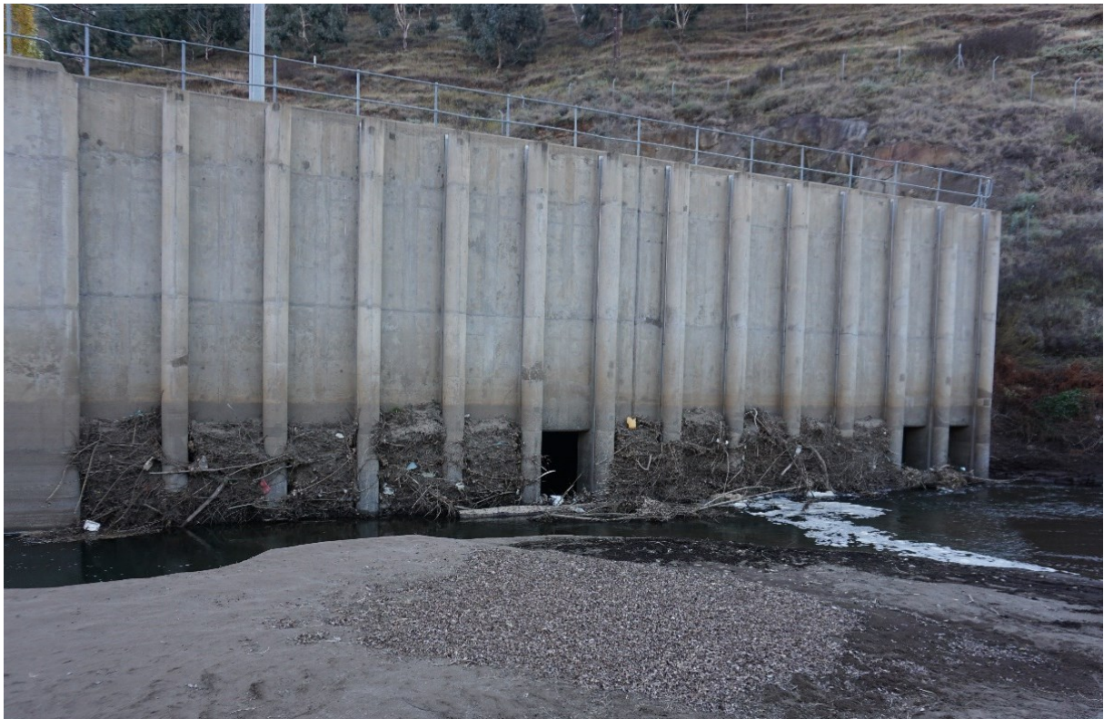
Figure 3. Blinding of the screens at Matsoku Weir (7 June 2022)
