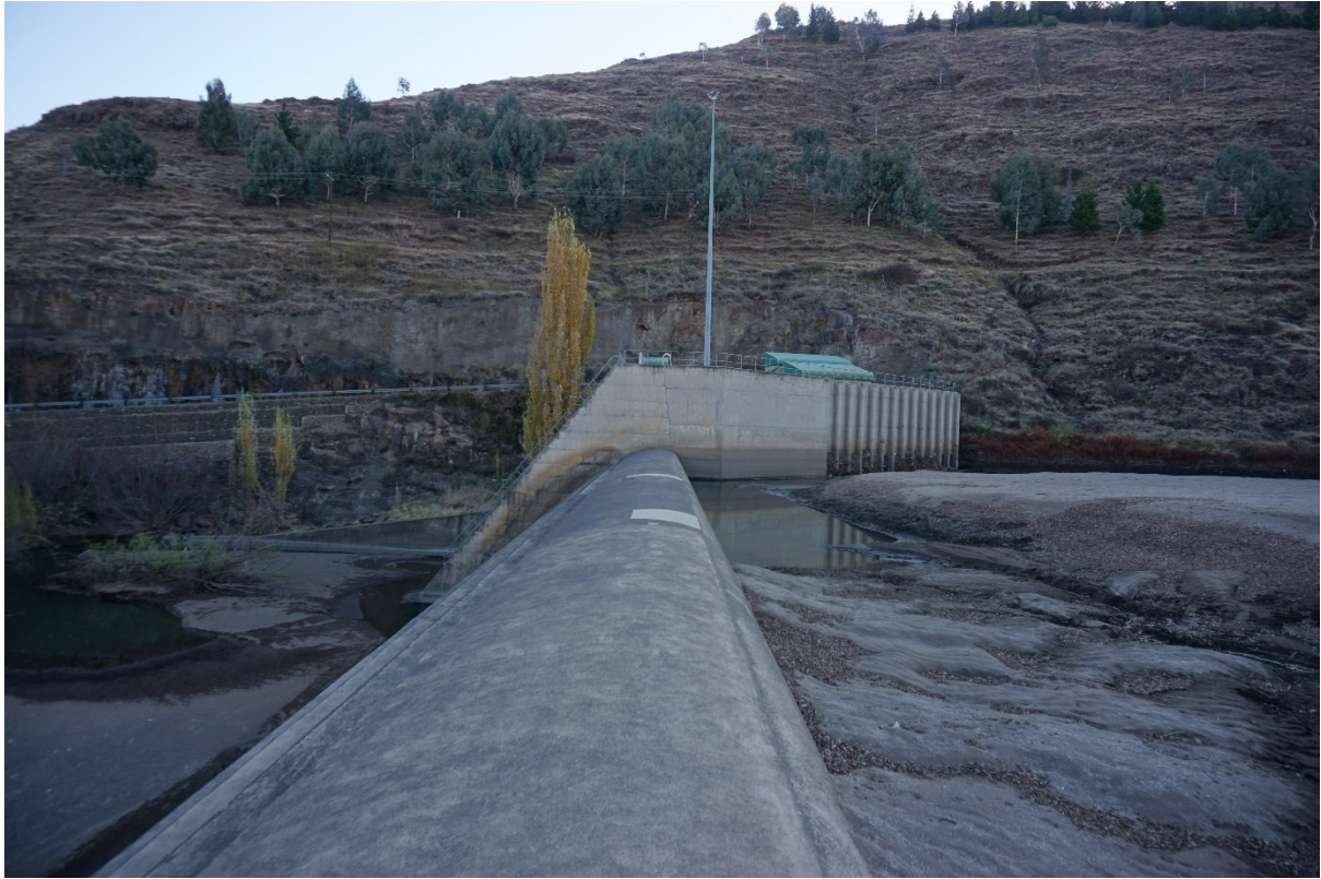
Figure 5. The Matsoku weir and divergence tunnel as viewed from the weir. The intake structure sits on the right bank of the Matsoku river. Water either enters the intake structure to flow to the Katse Dam or it spills over the weir.
