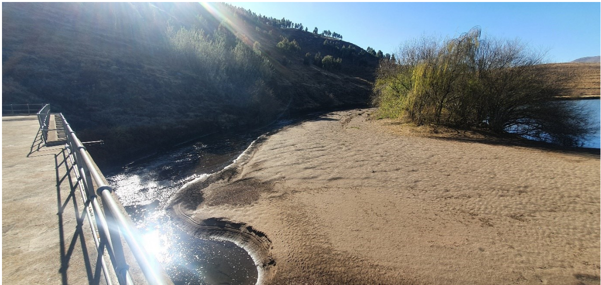
Figure 17. Sediment buildup in the river in front of the screens. The upstream end of the river can be seen towards the centre of the photo.
